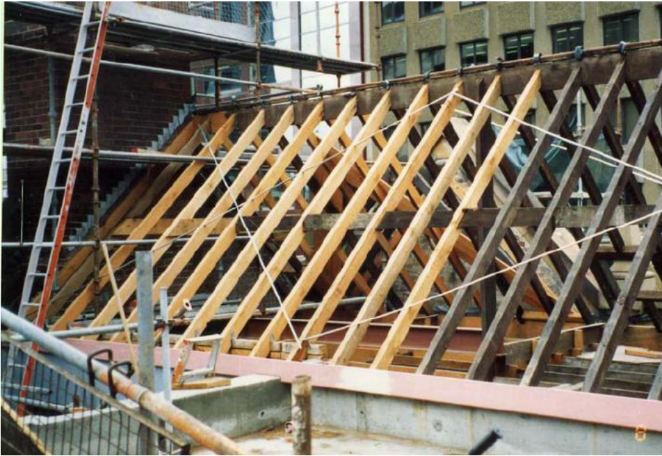
Figure 80 – Rebuilding of the roof to the George Street frontage of the Johnson’s building
