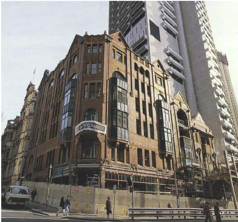
Figure 77 – Restoration of the Edwardian building facades. Note the scaffolding erected in front of the Commercial and Brooklyn Hotel buildings. The awning has also been removed.
