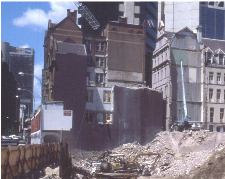
Figure 71 – View south to the building group showing the Brooklyn Hotel partially demolished (1983).
