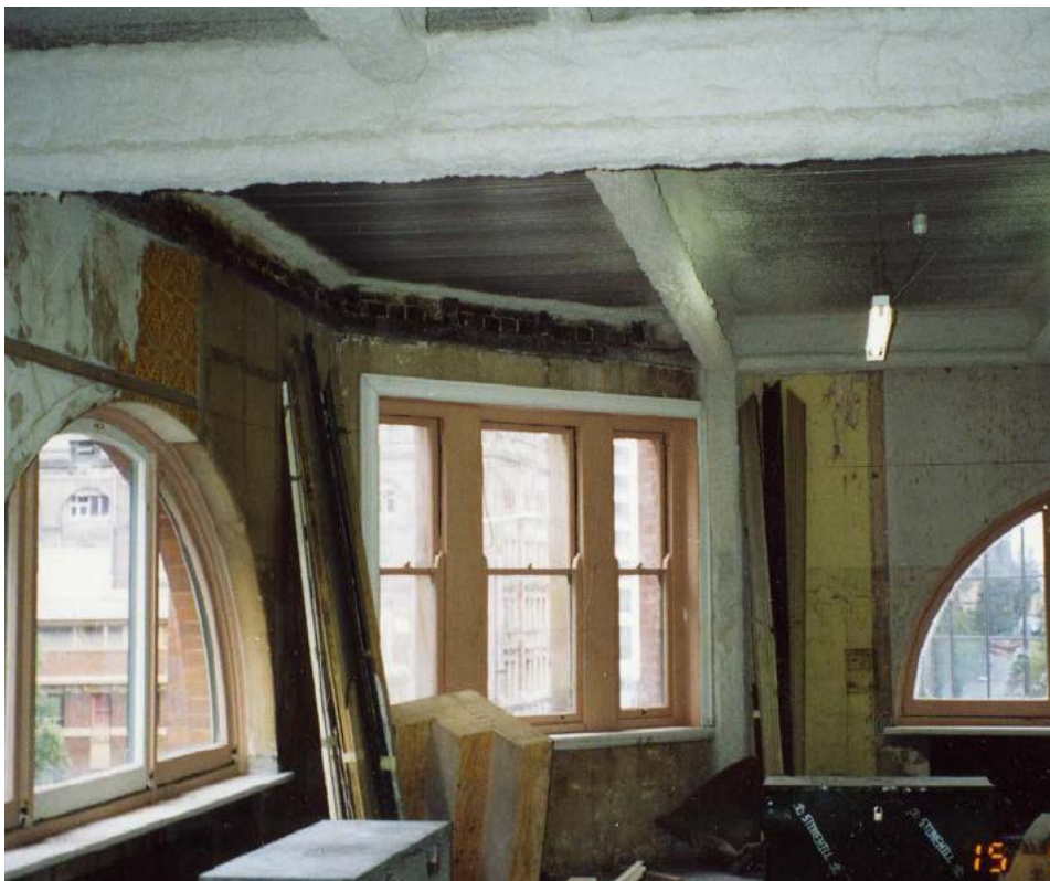
Figure 81 – View of internal works including fire rating- probably on the fifth floor of the Johnson’s Building.
