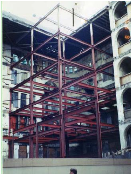
Figure 78– View of the girder structure within the corner Johnson’s Building. All floors have been demolished. (8/8/1990)
