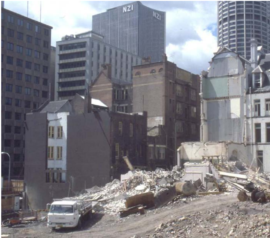
Figure 70 – The rear of the Johnsons group, with the Brooklyn Hotel shown at left and partially demolished Royal Naval House at right. (1983)
