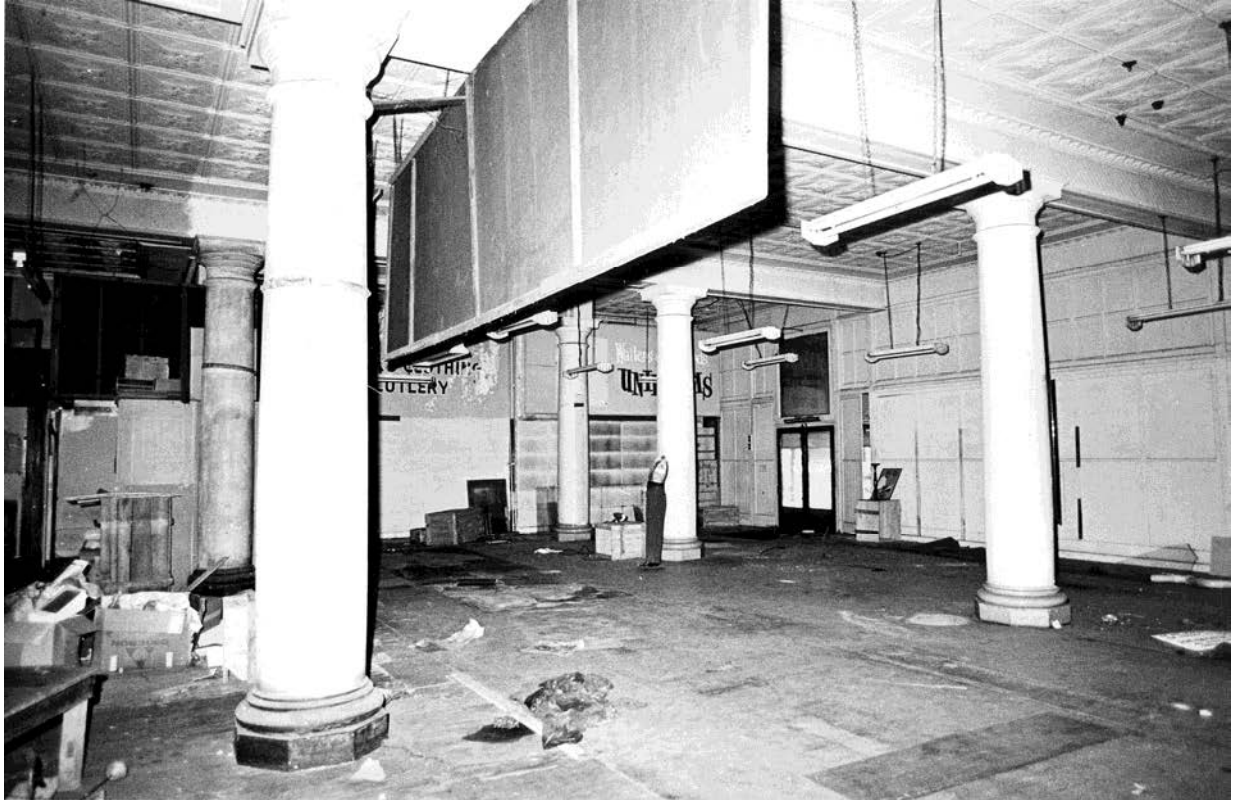
Figure 67 – The former ground floor interior of the Johnsons building, shown vacant. The original second entry to George Street is shown, along with original internal finishes.
