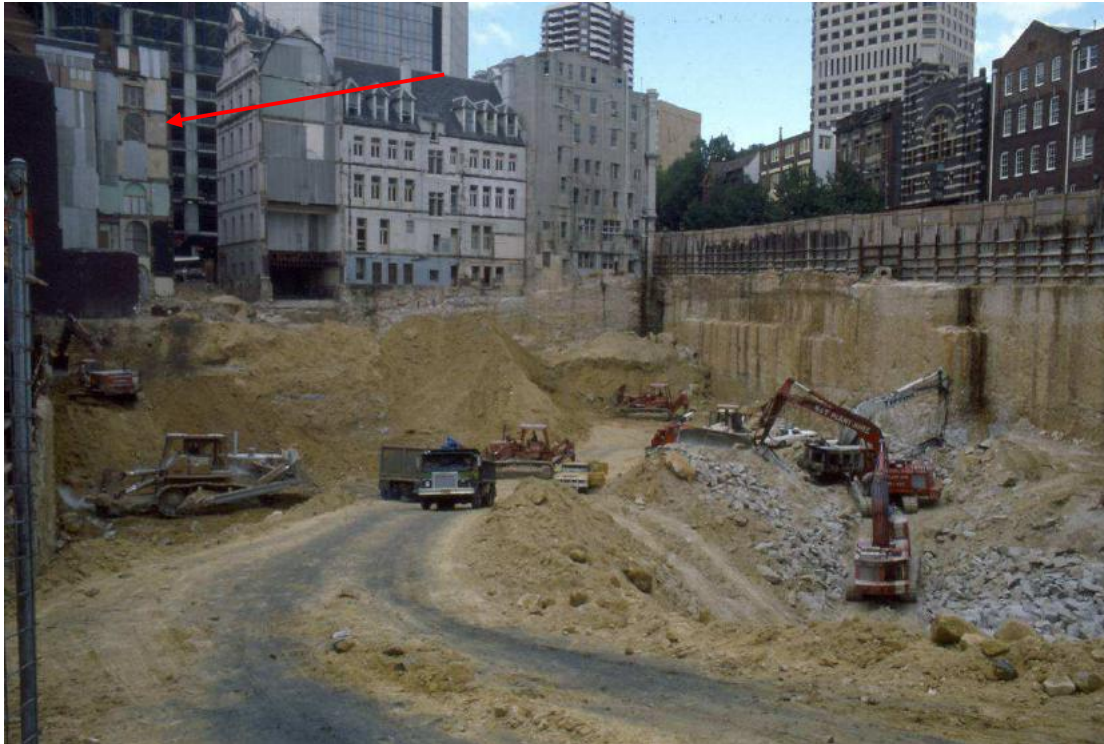
Figure 74 – The rear of the Johnson’s Building during the demolition and excavation (1984). The rear wings of The Brooklyn Hotel and the Commercial Building have been demolished, along with part of the Johnson’s Building (indicated). The form of the arched openings are retained in the stair well (refer views of the existing stair shown in section 3.4), though they have been infilled.
