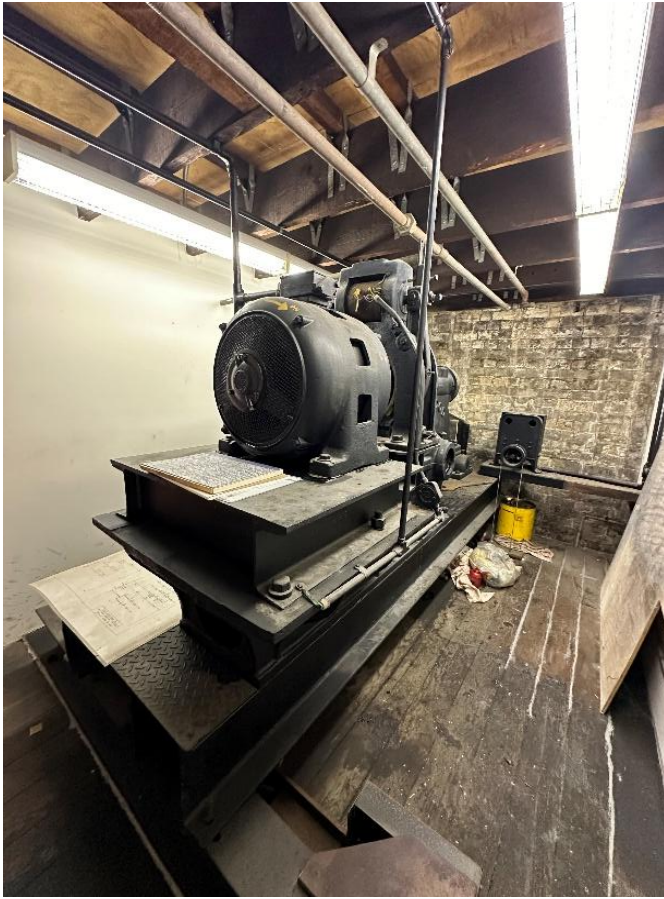
Figure 101: The lift room on mezzanine floor above Level 3. (Source: PMNSW 2026)
