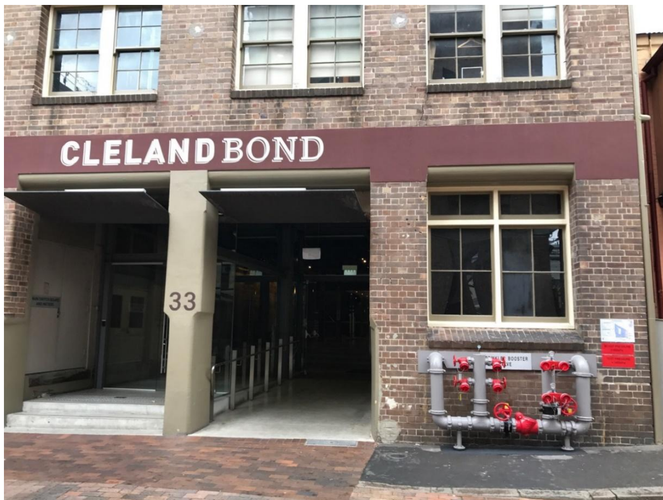
Figure 36: New booster system adjoining the main entrance to Cleland Bond Store, 2021. (Source: Gartner Rose gartnerrose.com.au )
