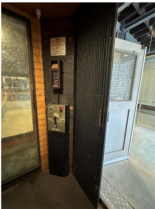
Figure 99: The original lift control panels.
