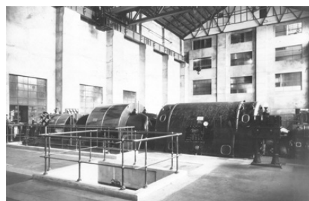
Figure 2.7.100 Parsons 22,000 kW Turbo Alternator installed (No. 9), 1926 (Design 5 collection).
