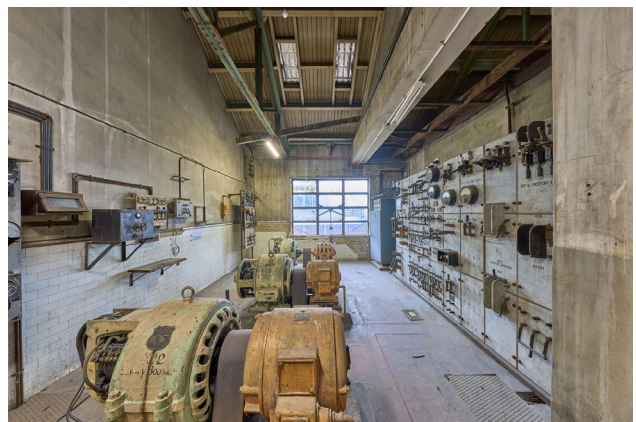
Figure 6.6.44 Motor Generator Room on Level 3 of the Switch House, 2023 (courtesy of Chris Bennett: Evolving Picture).
