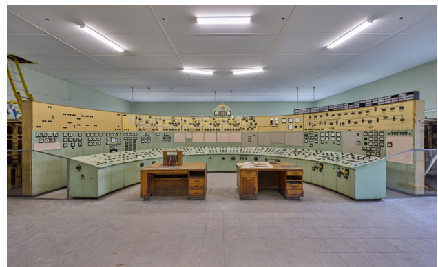
Figure 3.2.35 Control Room Interior, November 2023 (courtesy of Chris Bennett: Evolving Picture).
