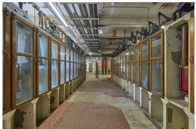
Figure 6.6.48 Extant 25 Cycle Switches on Level 2 of the Switch House, 2023 (courtesy of Chris Bennett: Evolving Picture).
