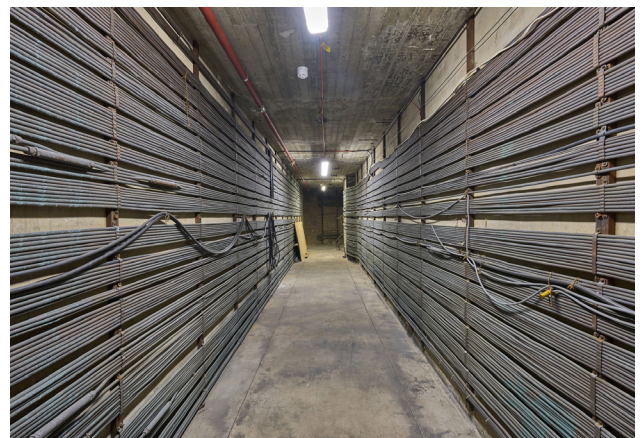
Figure 3.5.6 Cable Room in Control Room Building, July 2024 (courtesy of Chris Bennett: Evolving Picture).
