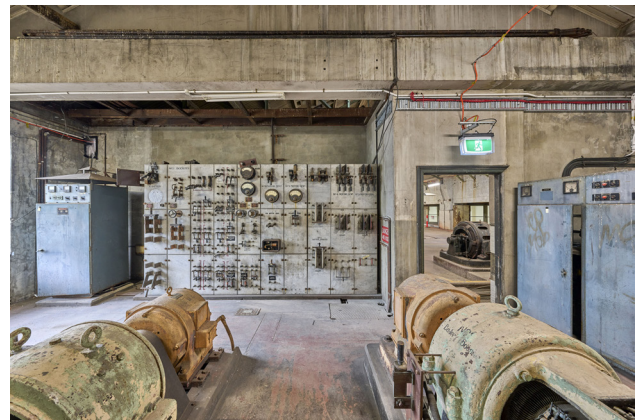
Figure 6.6.6 Motor Generator Room with a myriad of extant machinery and equipment, 2023 (courtesy of Chris Bennett: Evolving Picture).
