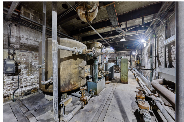
Figure 6.6.27 Dense configuration of tanks and pipework on the north, mezzanine level of the Pump House, 2023 (courtesy of Chris Bennett: Evolving Picture).
