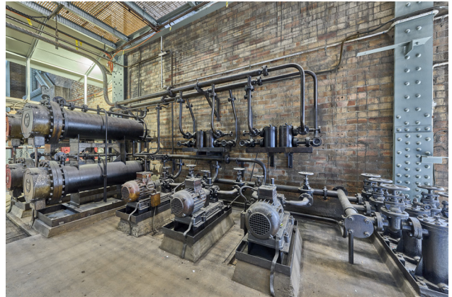
Figure 6.6.8 Smaller miscellaneous machinery on Level 1 of the Boiler House, 2024 (courtesy of Chris Bennett: Evolving Picture).
