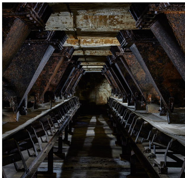
Figure 6.6.12 Coal Handling Shed basement conveyors, 2024 (courtesy of Toby Peet).
