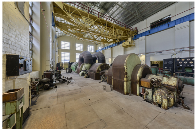
Figure 2.2.33 Turbine Hall No. 1 Turbo-Alternator with Overhead Crane above, 2024 (courtesy of Chris Bennett: Evolving Picture).
