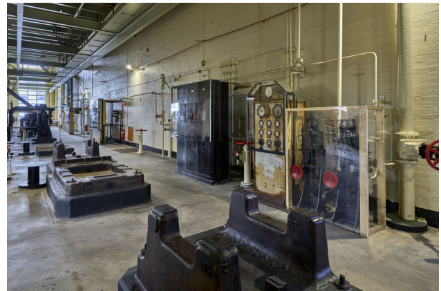
Figure 2.2.13 Northern half of the Pump House, Level 2, with the extant equipment and machinery of the Feedwater System, 2024 (courtesy of Toby Peet).
