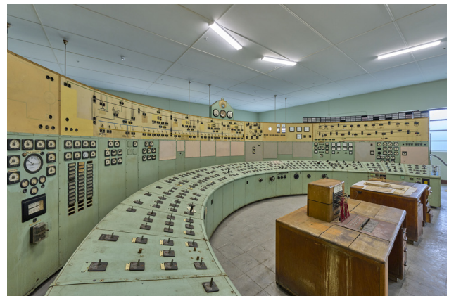
Figure 2.2.26 Control Room, 2023 (courtesy of Chris Bennett: Evolving Picture).
