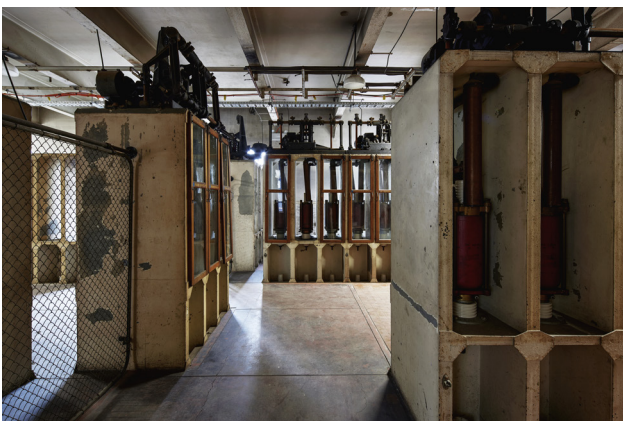
Figure 6.19.1 Switch House Cycle Switches, 2024 (courtesy of Toby Peet).
