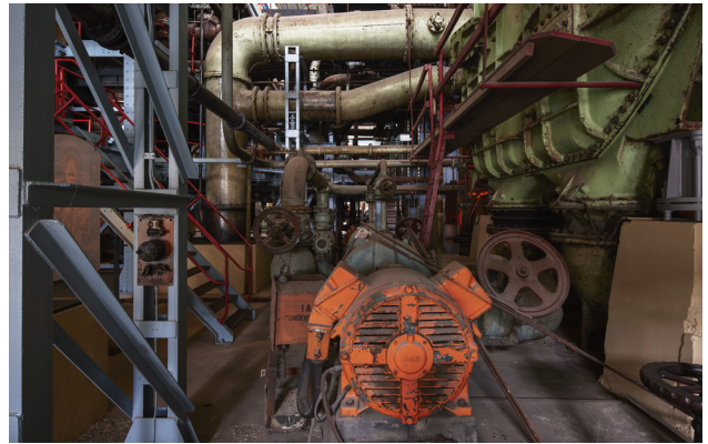
Figure 6.20.2 Dense configuration of machinery at the north end of the Turbine Hall Ground Level, 2024 (courtesy of Toby Peet).
