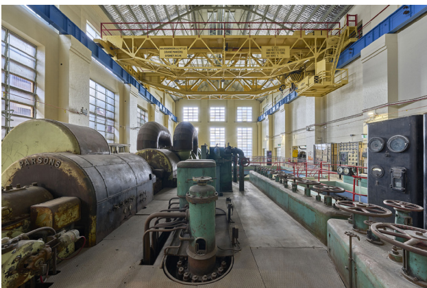
Figure 6.6.30 North end of the Turbine Hall with the Parsons Turbo-Alternator Set and other machinery and equipment, 2024 (courtesy of Chris Bennett: Evolving Picture).
