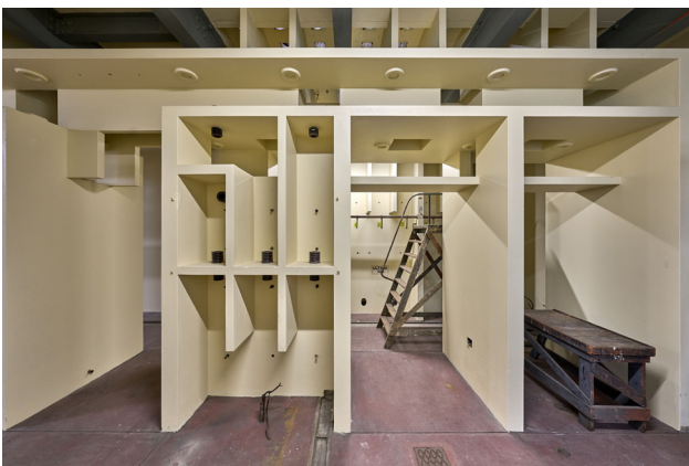
Figure 6.6.52 Level 1 concrete housing for the bus bars, 2023 (courtesy of Chris Bennett: Evolving Picture).
