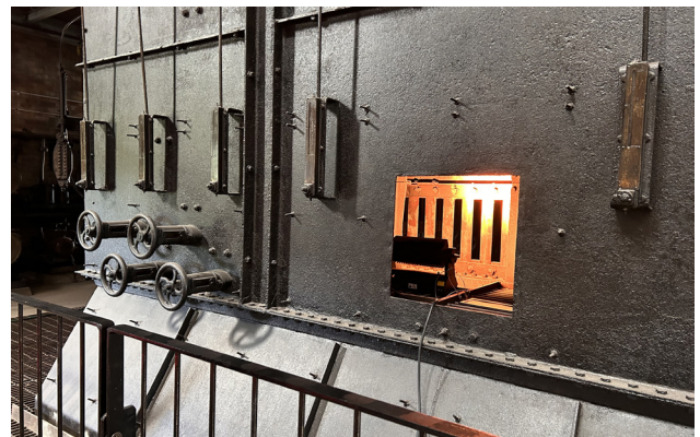
Figure 6.13.2 Interpretative lighting on the inside of the No. 1 Boiler, 2024 (Design 5 – Architects).
