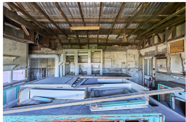
Figure 6.6.39 Laboratory on Level 4, 2024 (courtesy of Chris Bennett: Evolving Picture).
