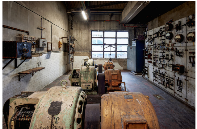
Figure 4.2.39 Motor Generator Room in the Switch House, 2024 (courtesy of Toby Peet).
