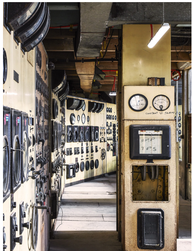
Figure 3.2.20 Boiler House Control Room, 2023 (courtesy of Toby Peet).
