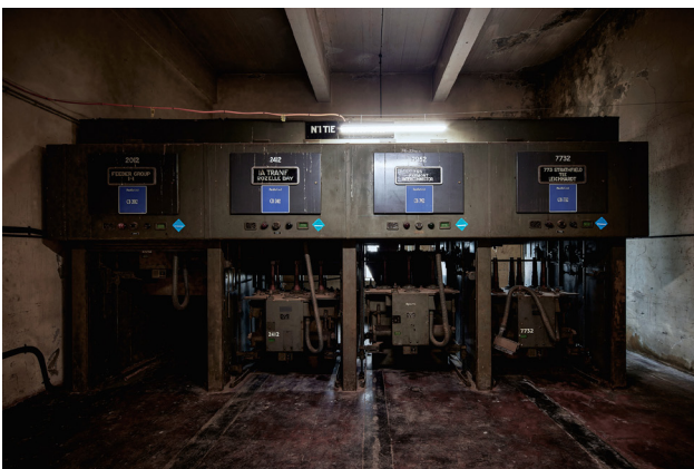
Figure 6.6.47 The No. 1 Tie Bank on Level 2 of the Switch House, 2024 (courtesy of Toby Peet).
