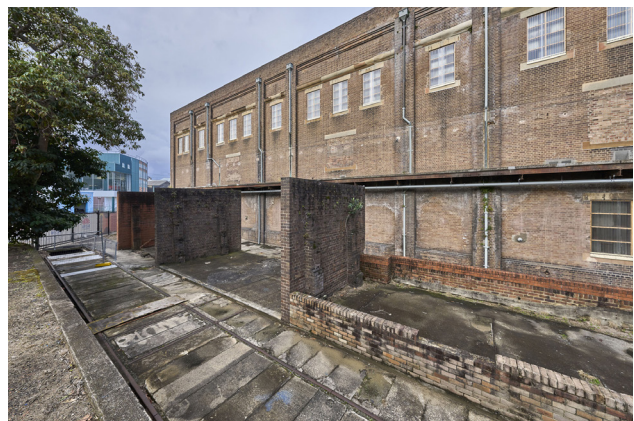
Figure 6.11.5 Transformer Yard, 2024 (courtesy of Chris Bennett: Evolving Picture).
