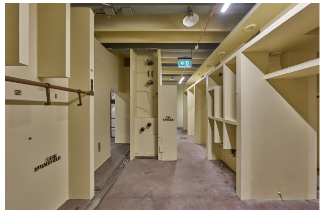
Figure 5.10.1 Bus bars space on Level 1 of the Control Room Building, 2024. This space would impose design and BCA upgrade challenges in reuse application. (courtesy of Chris Bennett: Evolving Picture).
