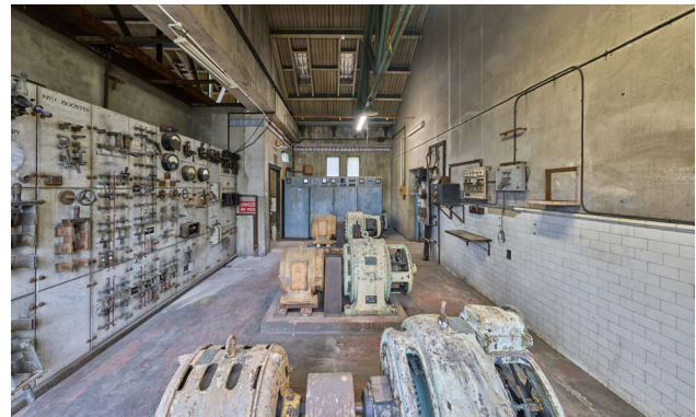
Figure 3.2.32 Switch House Motor Generator Switch Room, November 2023 (courtesy of Chris Bennett: Evolving Picture).
