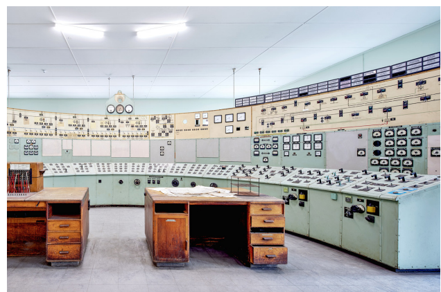
Figure 6.6.50 The Control Panel of the 1948 Control Room, 2024 (courtesy of Toby Peet).
