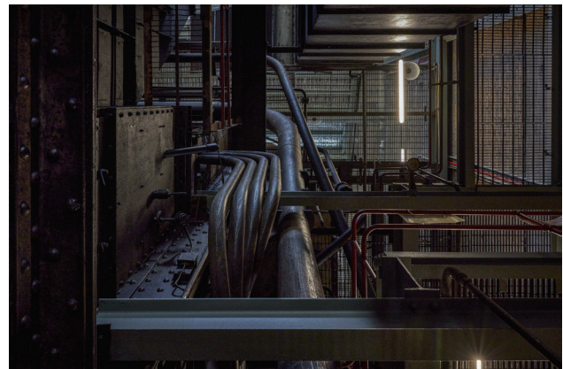
Figure 6.6.19 Inside of the extant Babcock and Wilcox No. 1 Boiler, 2023 (courtesy of Toby Peet).
