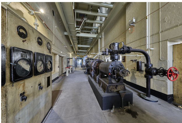
Figure 2.2.32 Pump House High Pressure Feedwater Pumps, 2024 (courtesy of Chris Bennett: Evolving Picture).
