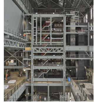
Figure 4.2.2 No. 1 Boiler, 2024 (courtesy of Chris Bennett: Evolving Picture).
