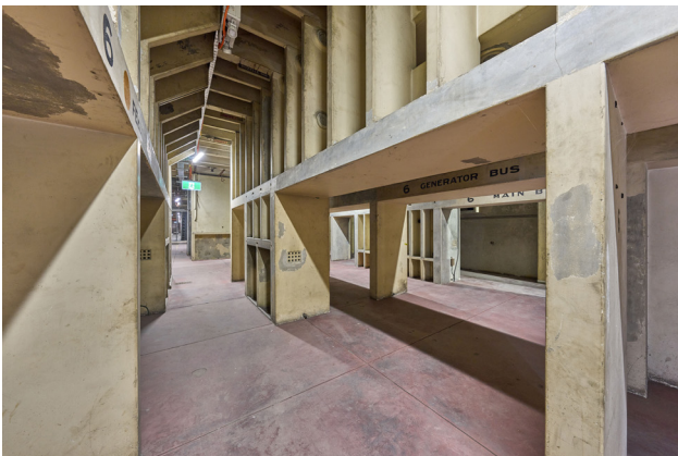
Figure 6.6.42 South end of Level 1 of the Switch House with the extant concrete cable runs, 2023 (courtesy of Chris Bennett: Evolving Picture).
