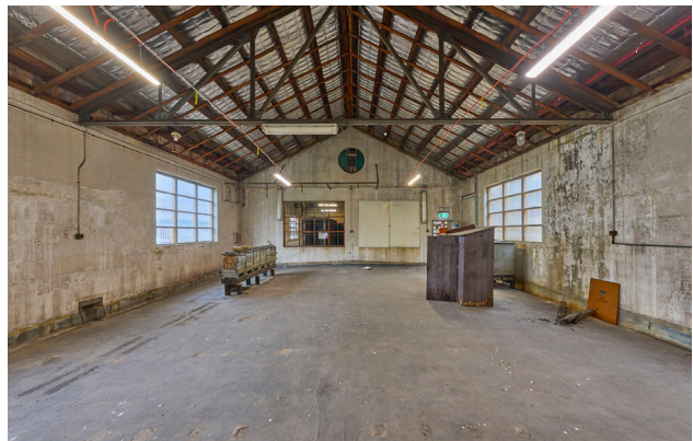
Figure 7.11 Switch House Level 3 battery room, 2024 (courtesy of Chris Bennett: Evolving Picture)
