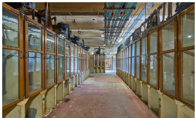
Figure 7.10 Switch House Level 2 cycle switches, 2024 (courtesy of Chris Bennett: Evolving Picture)
