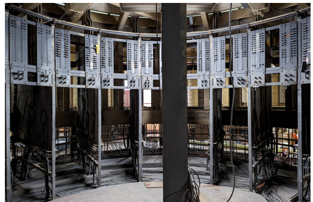
Figure 8.5 First Floor Cable Room, 2024 (Design 5 - Architects)
