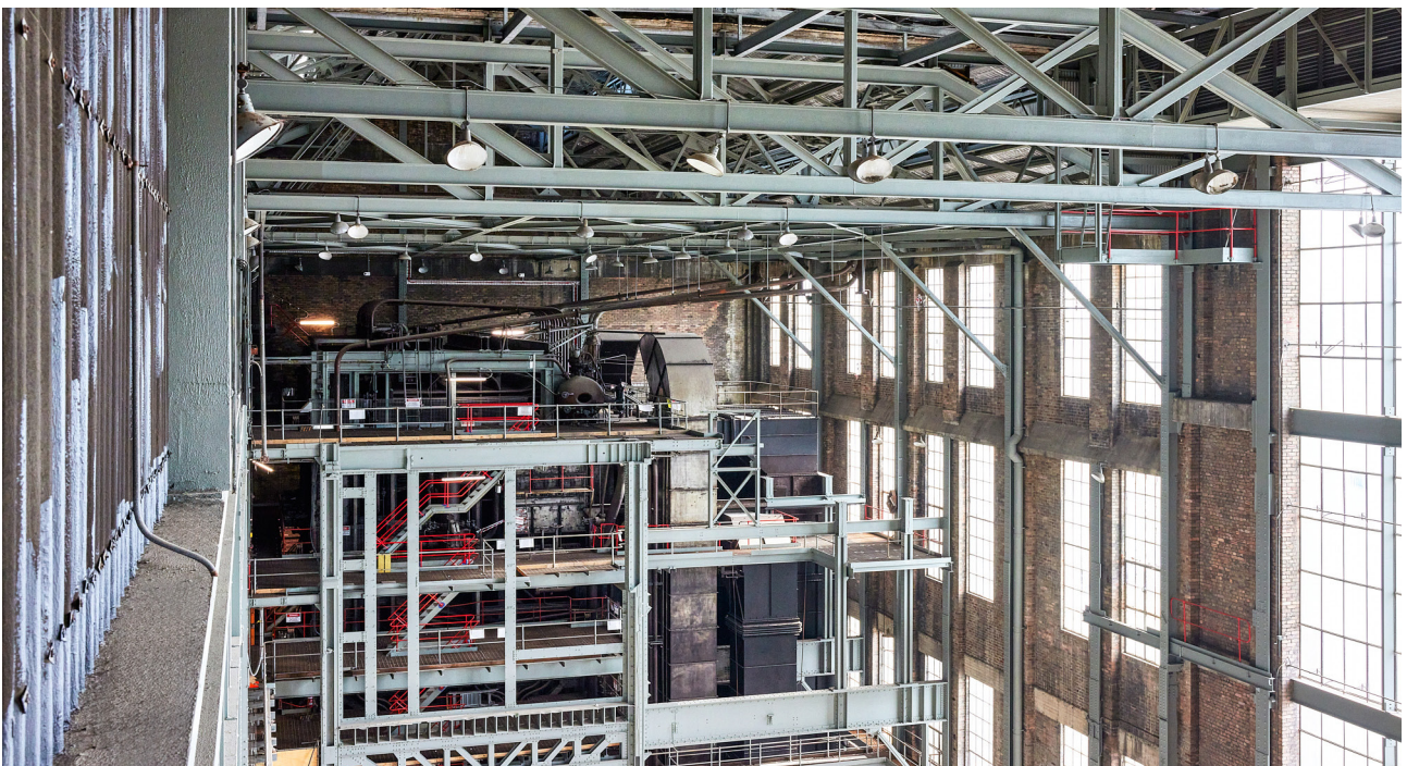
Figure 3.6 Extant Boiler No. 1, 2024 (courtesy of Toby Peet)
