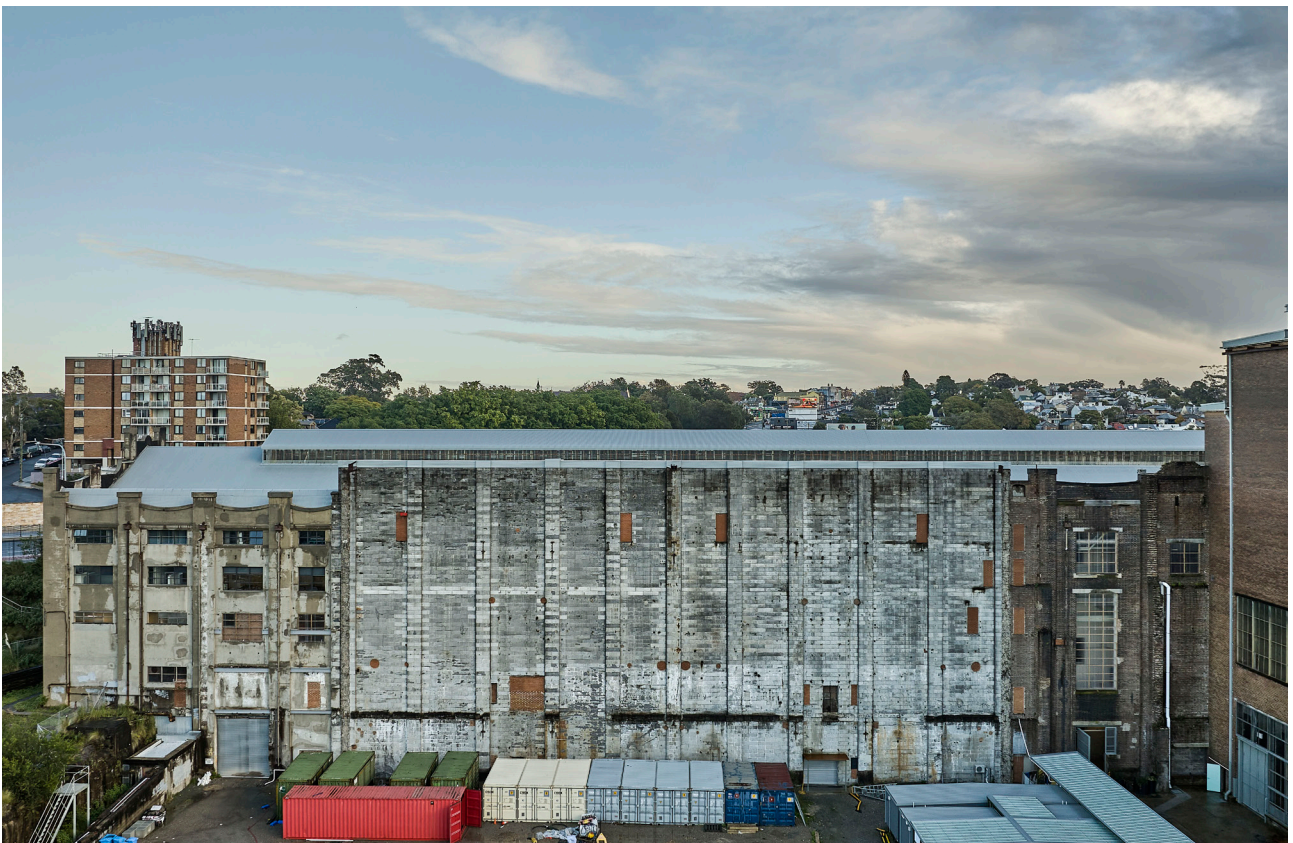
Figure 4.7 Pump House East Elevation, between Administration and Staff Building (left) and Boiler House (right), 2024 (courtesy of Chris Bennett: Evolving Picture)
