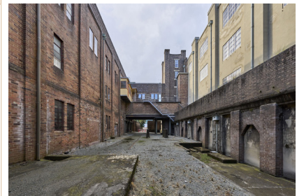
View of the South West Yard looking north towards the Control Room bridge, 2024 (courtesy of Chris Bennett: Evolving Picture)
