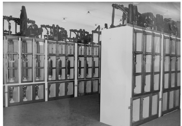
Figure 8.9 Second Floor Switch Floor (CS2.2) with oil circuit-breakers, 1951 (courtesy of Department of Railway Archive, E2603)
