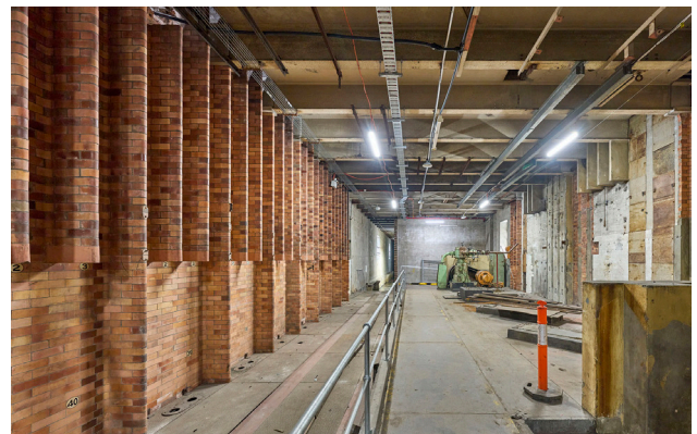
Figure 7.5 Switch House Ground Floor, SH G.5 looking north, 2024 (courtesy of Chris Bennett: Evolving Picture)
