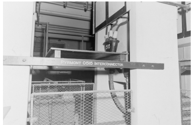
Figure 7.8 Switch House Level 1 cable groups, 1957 (courtesy of ECNSW Archive, 01029 White Bay 1)
