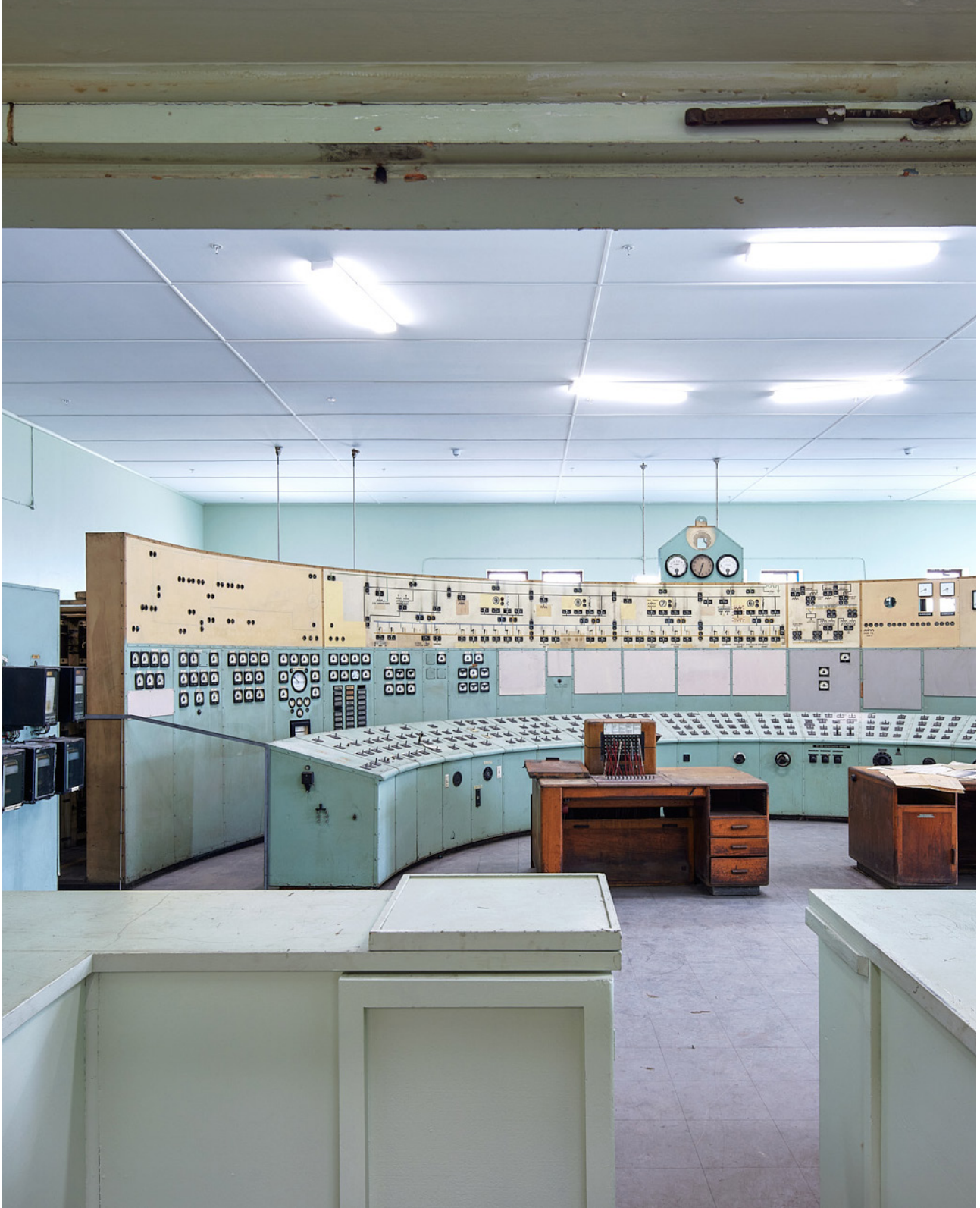
Figure 8.1 Control Room, 2024 (courtesy of Toby Peet)
