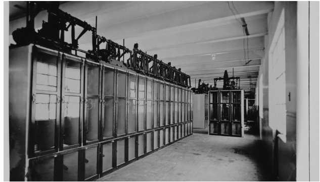
Figure 7.9 Switch House Level 2 cycle switches, date unknown, pre-1950s (courtesy of Railway Department Archive Photo Cards, 1693-105)
