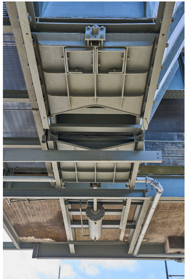
Figure 2.7 Ash Handling Tower under the drums, 2024 (courtesy of Chris Bennett: Evolving Picture)
