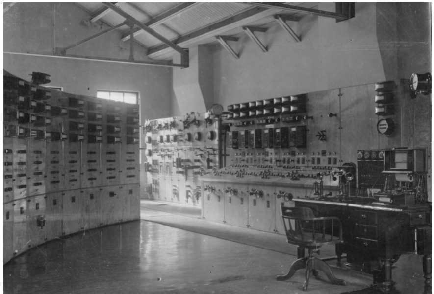
Figure 2.5 White Bay Power Station. The original Control Room at the south end of the turbine hall.
