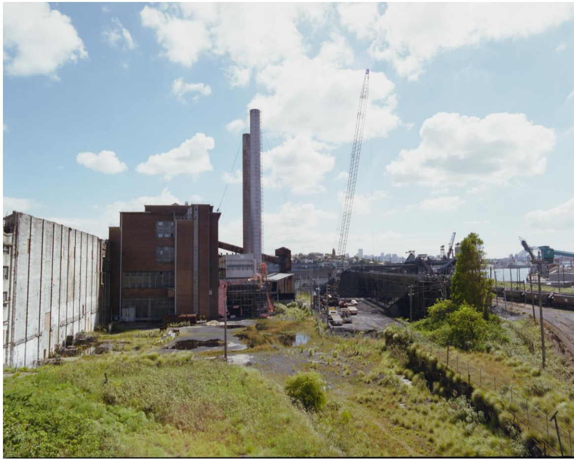
Fig 59: View over South Yard, 1990. Precipitators under demolition in Coal Loader plaza. (Archives NSW, NRS-20347-1 cn70015 L)
