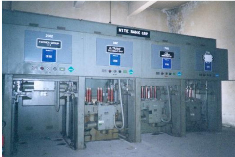
No. 1 Tie Bank Group
