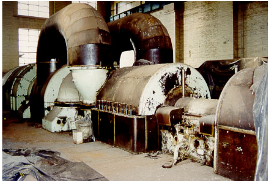
Figure 3.5 Parsons turbo-alternator, located in the southern end of the Turbine Hall. The turbo-alternators are integral to the Power Generating System.
