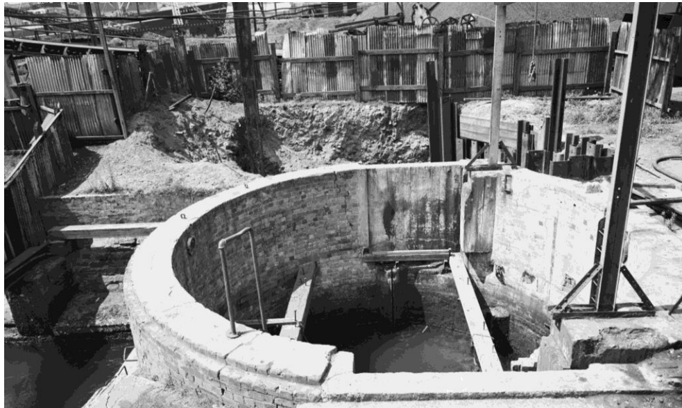
Fig 21: White Bay northern penstock modifications, Water Circulating Conduit (to White Bay), 1957. (NSW Archives, NRS 20347-1 1031 A)
