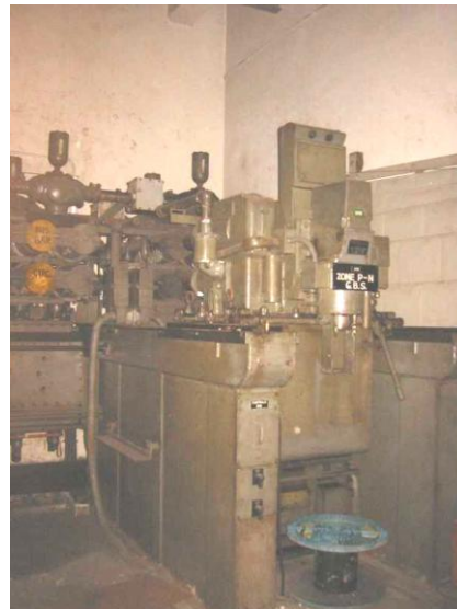
Bus Bar Circuit Breaker
